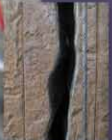
Variable crack widths
