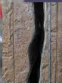
Variable crack widths
